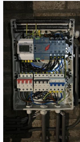
Rode schakelaar in de off-grid kast.
